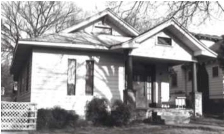
1998 – main house at 705. Unpermitted changes since 1978 include replacement of front window with two smaller windows, and enclosure of the previously exposed rafter tails.
